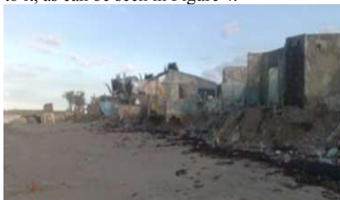
Figure 4. Image showing the damage caused by waves on the beach, which has damaged restaurants, homes, businesses, palapas, and streets in the community of Sánchez Magallanes, Tabasco.
